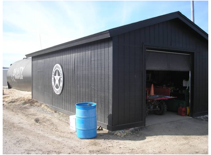
Photo #2 – View of a wellhouse/storage building observed adjacent to the northeast corner of the soccer fields.
