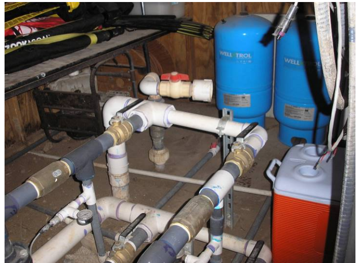
Photo #4 – View of assorted equipment associated with the water well within the wellhouse/storage room.
