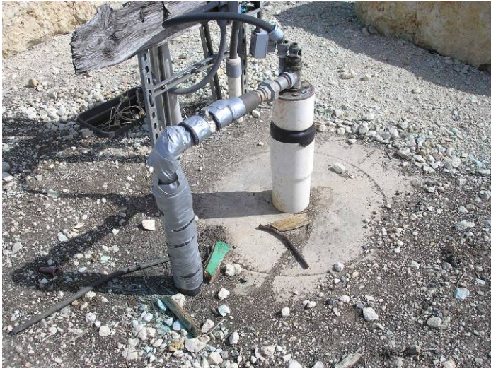
Photo #21 – View of PRF #S-7 observed in the eastern portion of the project site along the eastern perimeter of the on-site soccer fields.
