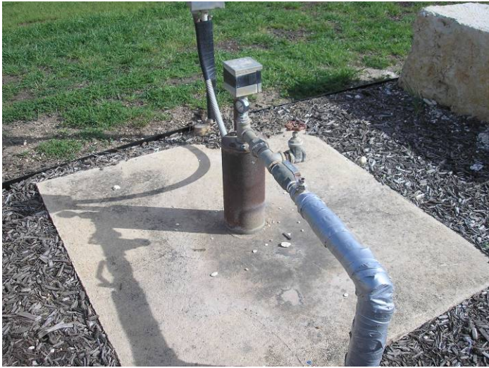
Photo #5 - View of PRF #S-2 located in the northern portion of the project site along the northern perimeter of the soccer fields
