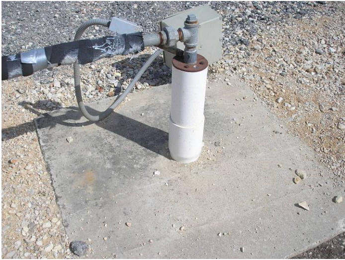
Photo #25 – View of PRF #S-8 observed in the eastern portion of the project site along the eastern perimeter of the on-site soccer fields.
